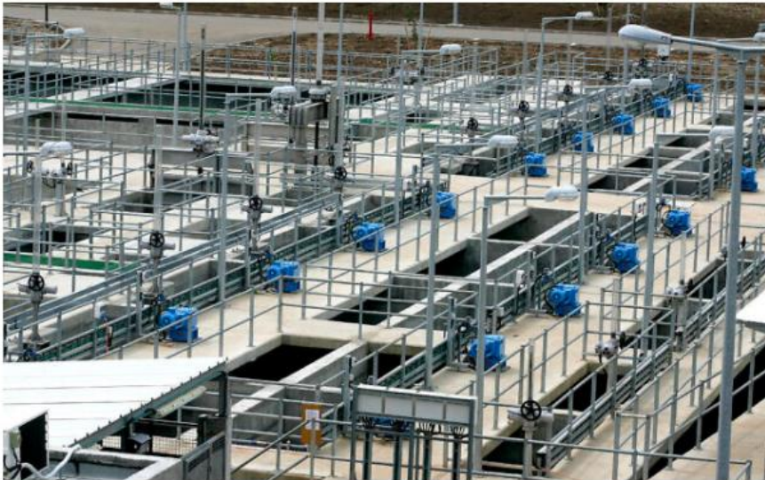
The Eshkol water filtration plant in northern Israel, April 17, 2007. (Moshe Shai/FLASH90)
